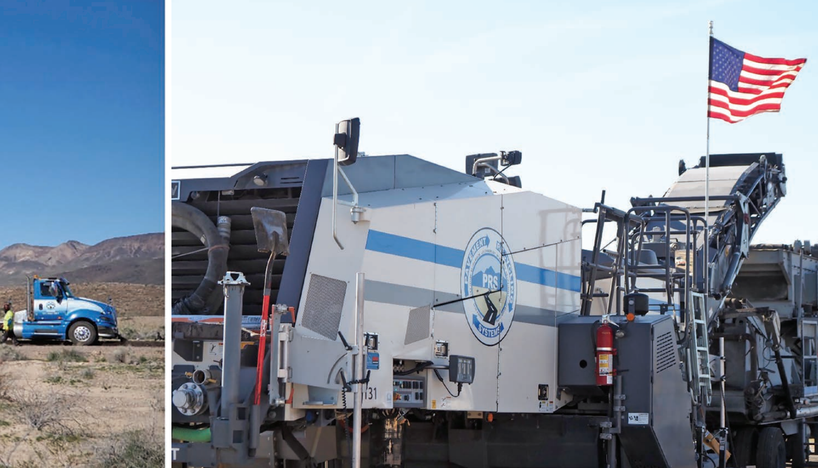
Above: Pavement Recycling Systems' Wirtgen 380 CRi full-lane (12.5 feet) milling machine grinding and conveying existing RAP material into the recycling unit.
